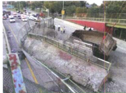
After a bridge strike—Waterbury Avenue Bridge in the Bronx
